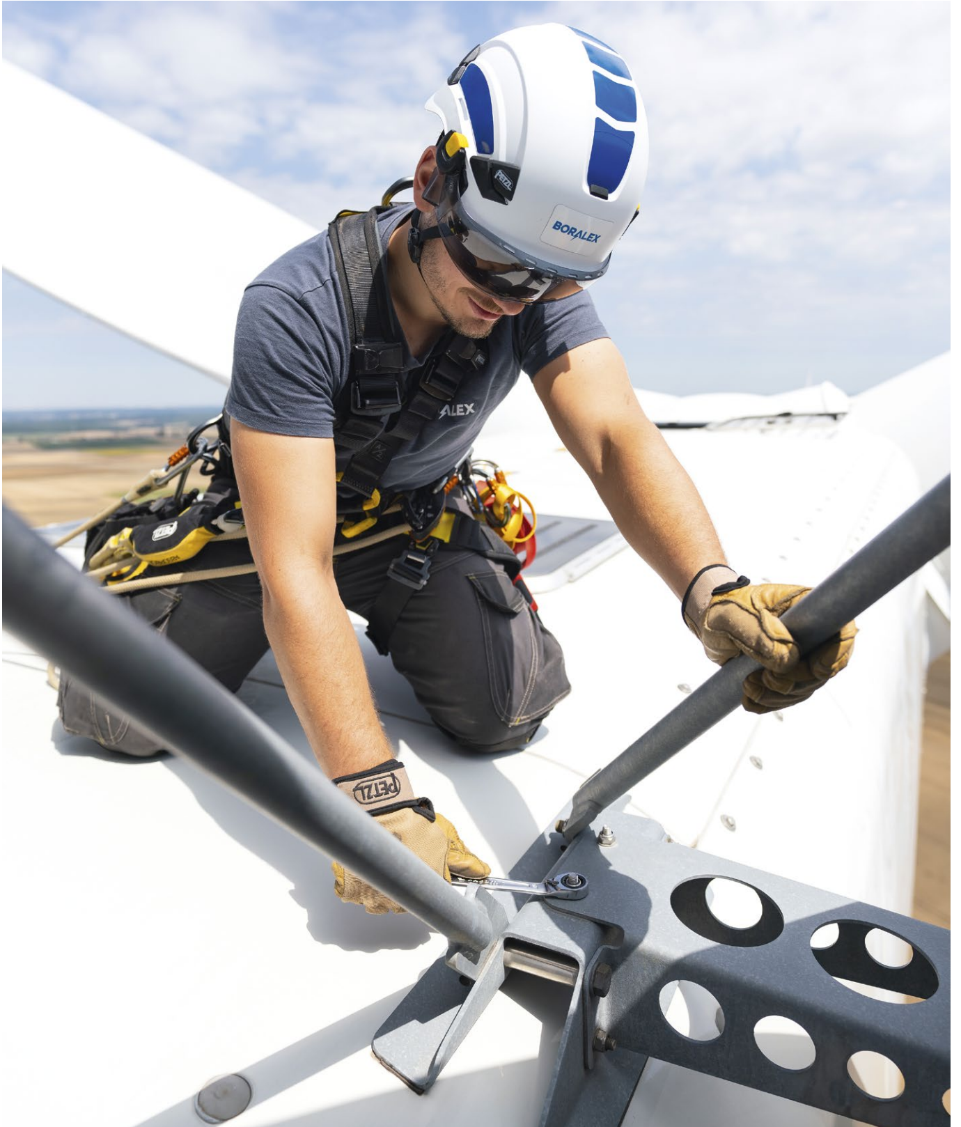
Maintenance and inspection of wind turbines in Vallée D'Arce, Champagne, France. © 2020 Petzl Distribution - Vuedici.org - Borealex SAS
