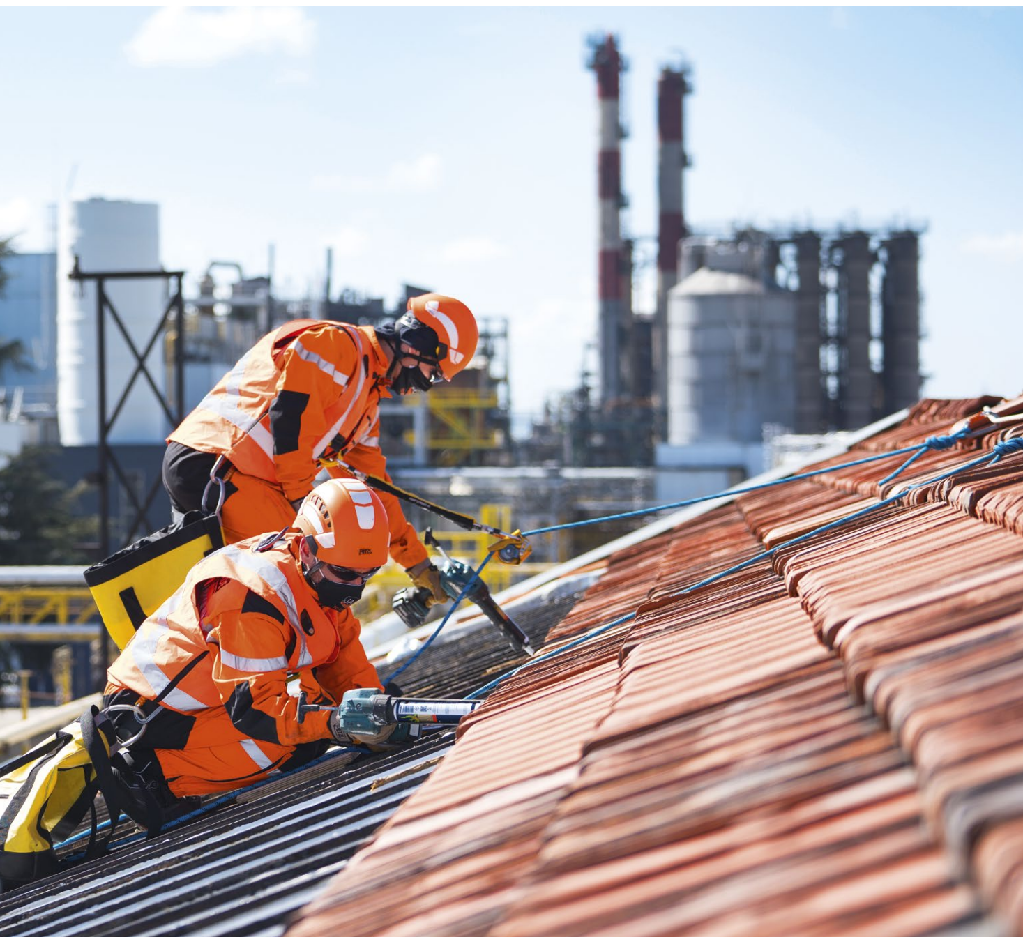
Industrial roof maintenance, Roussillon, France. © 2021 Petzl Distribution - Vuedici.org - JADE-SEGENS - Site de Roussillon
