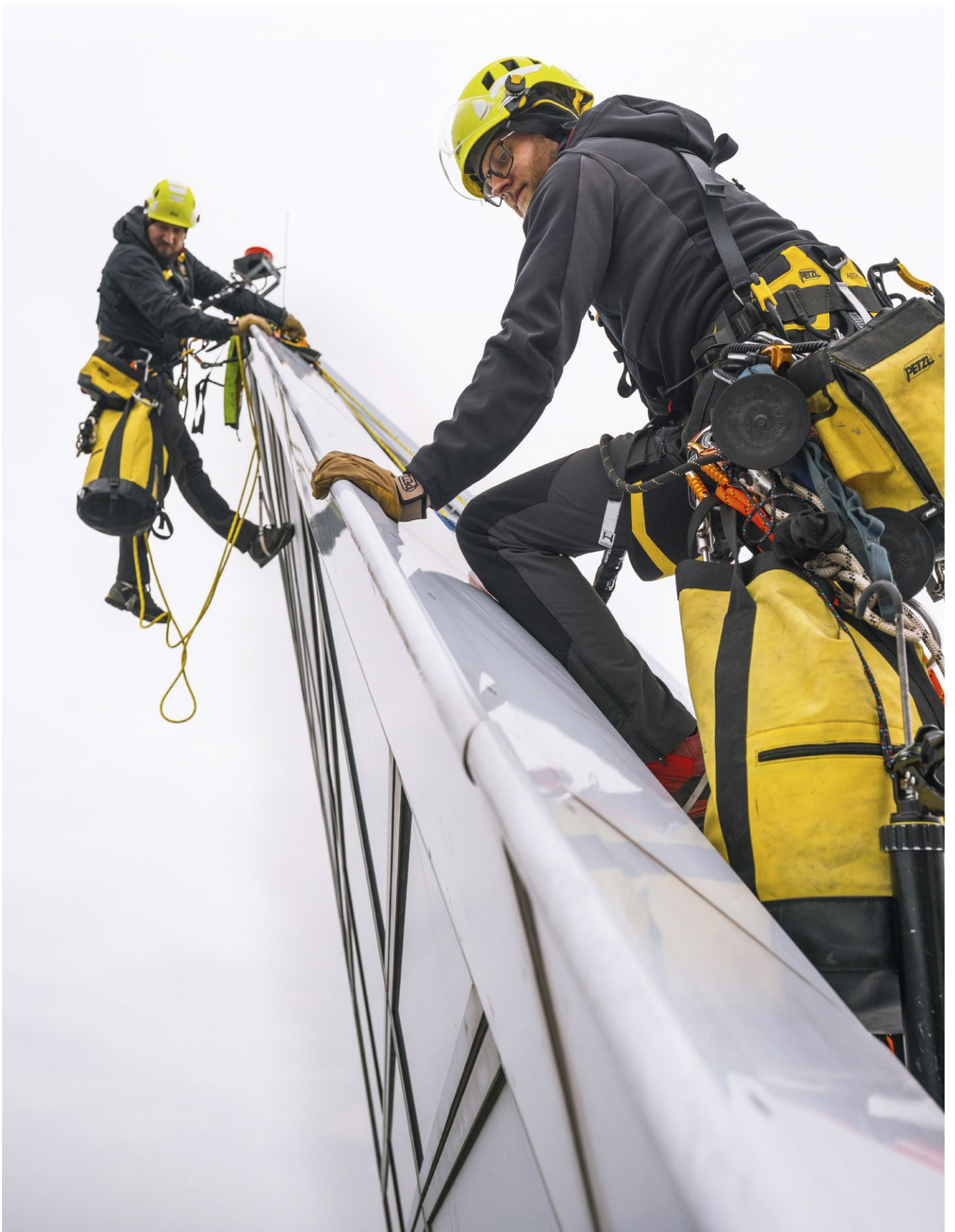
Glass panel maintenance at the Złota 44 tower, Warsaw, Poland. © 2020 Petzl Distribution - Vuedici.org - Topshelf - Złota 44
