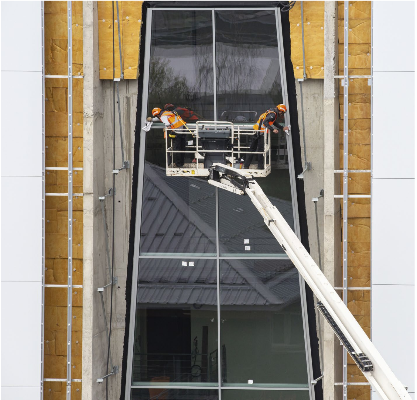
Glass window construction at the new Petzl testing facility, Croles, France. © Petzl Distribution - Lafouche
